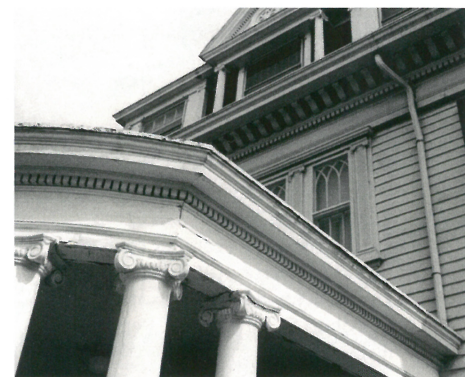
This residence shows a combination of brackets and dentils at the eaves of the main roof. A simpler dentil pattern is used at the porch roof, but the frieze area below it may have been more elaborate when the home was originally constructed. There is also a generous use of the Ionic capital, whether on the top of the porch columns or the pilasters on the window trim at the second floor or supporting the high gable eave on the upper floor.
