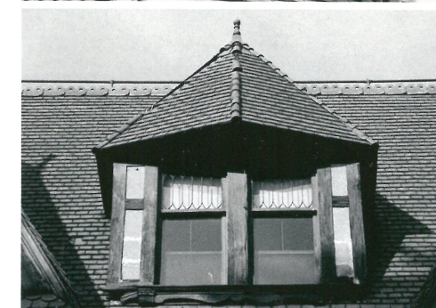
These photos show two different styles of dormers and camelbacks on the slate roof where the slope changes in direction.
