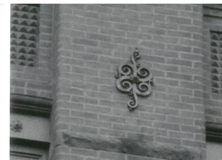
The photos at left show examples of decorative anchor plates. When a tall chimney or masonry wall becomes unstable or begins to buckle, a steel or iron tie rod was inserted through the wall to the interior framing. This rod is threaded through a turnbuckle and then tightened to pull the masonry wall tight to the structural framing. Sometimes a flat metal plate is placed on the exterior as a cap or something more decorative is used. Most anchor plates/tie rods in new construction are purely decorative as masonry construction has evolved.
